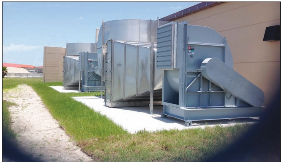
Exhaust Fans outside
