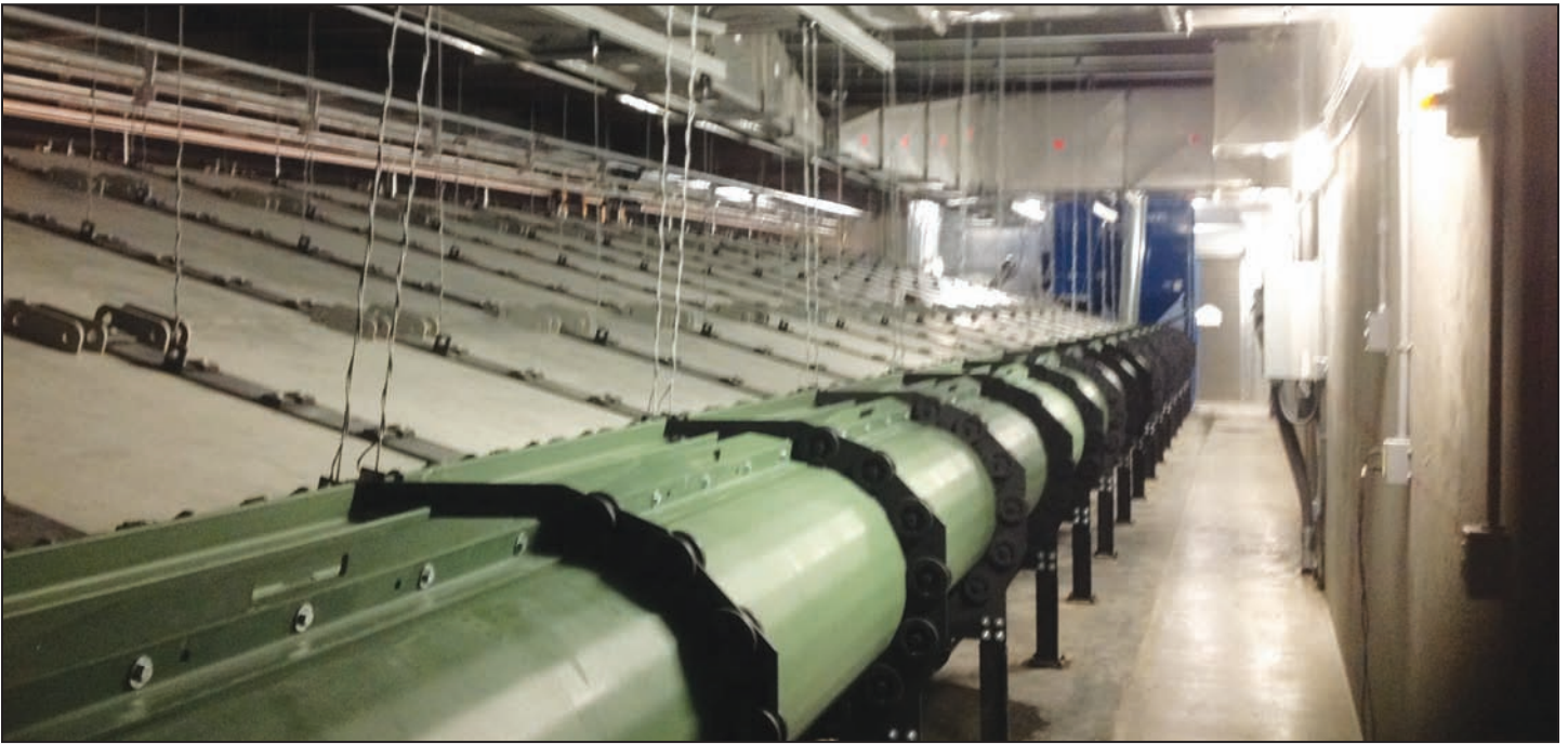
Exhaust duct at trap down range
